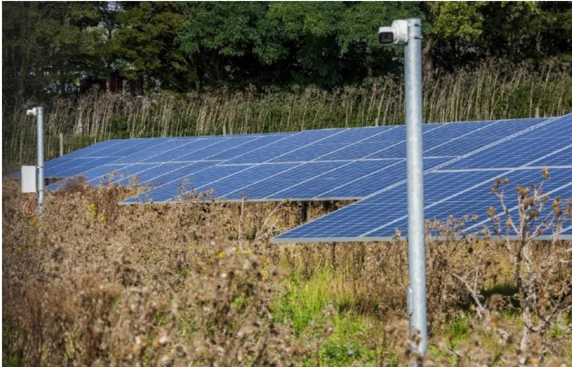
Image 4.15: Pole-mounted Security Camera (unpainted)
