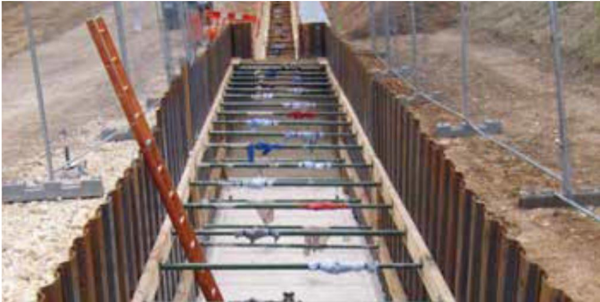
Image 4.11: Typical Joint Bay
