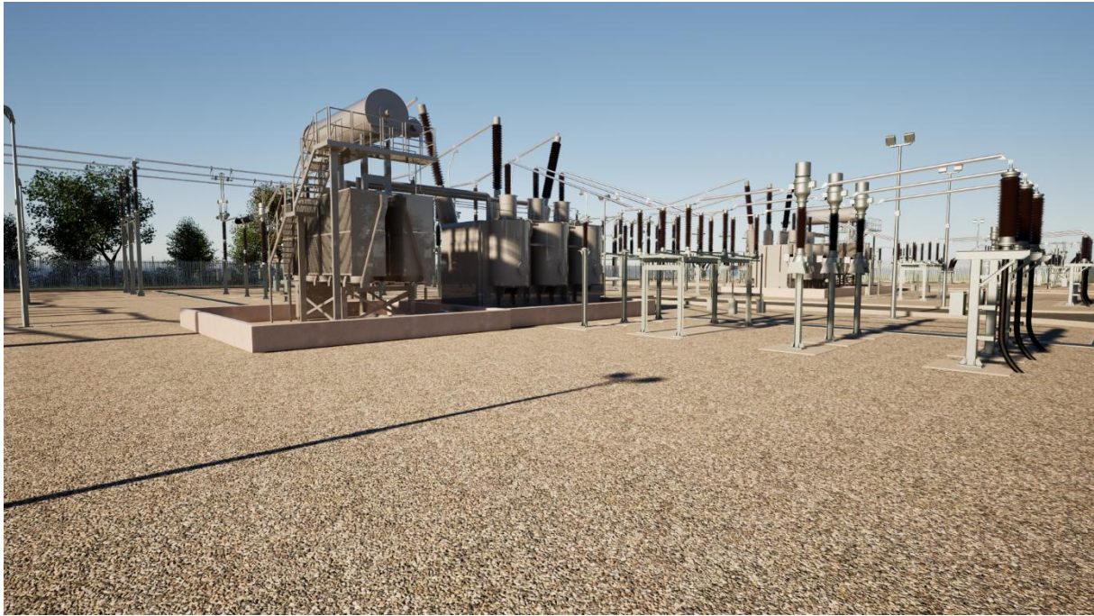
Image 4.9: Typical 400kV Power Transformer
