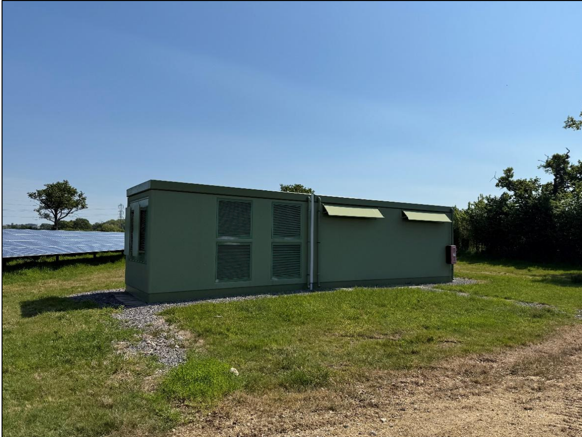
Image 4.6: Typical Conversion Unit / 33kV Sub-distribution Switch Room
