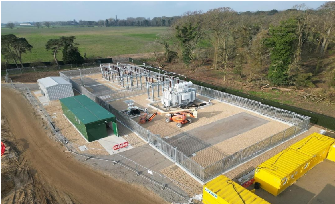
Image 4.8: 132/33kV Substation (Single Transformer)
