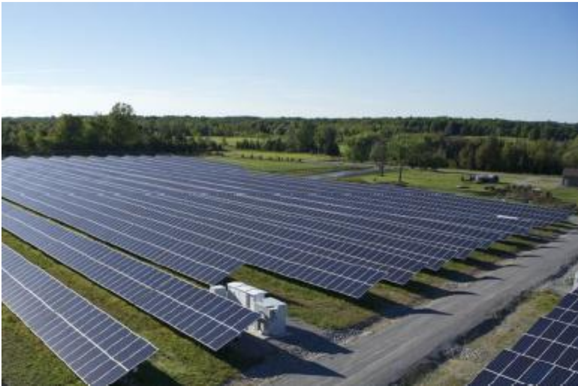
Image 4.2: Fixed South Facing PV Arrays
